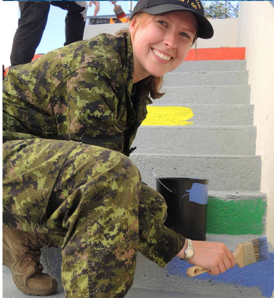
Major Rachel Middleton of Joint Task Force Pacific paints the staircase next to the Base Orderly Room as part of a painting project organized by the Defence Team Pride Advisory Organization. The stairs were painted in 11 different colours of the progressive rainbow flag on Aug. 23 in recognition of Public Service Pride Week. Photo: Peter Mallett/Lookout
